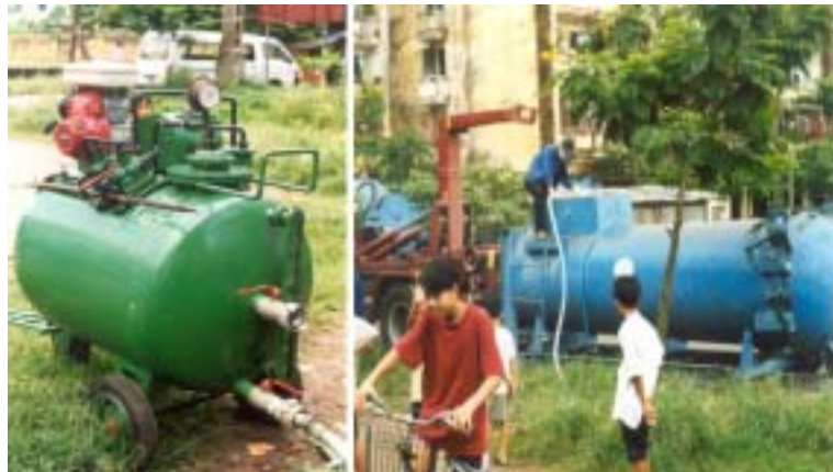
Figure 13: Mini-vacuum tug (350 L) for narrow lanes, used together with a intermediate-storage-tank placed in the next accessible road, Hai Phong, Vietnam.
